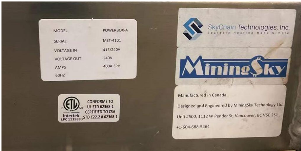
Picture above: PDU labels and stickers including ETL certification
