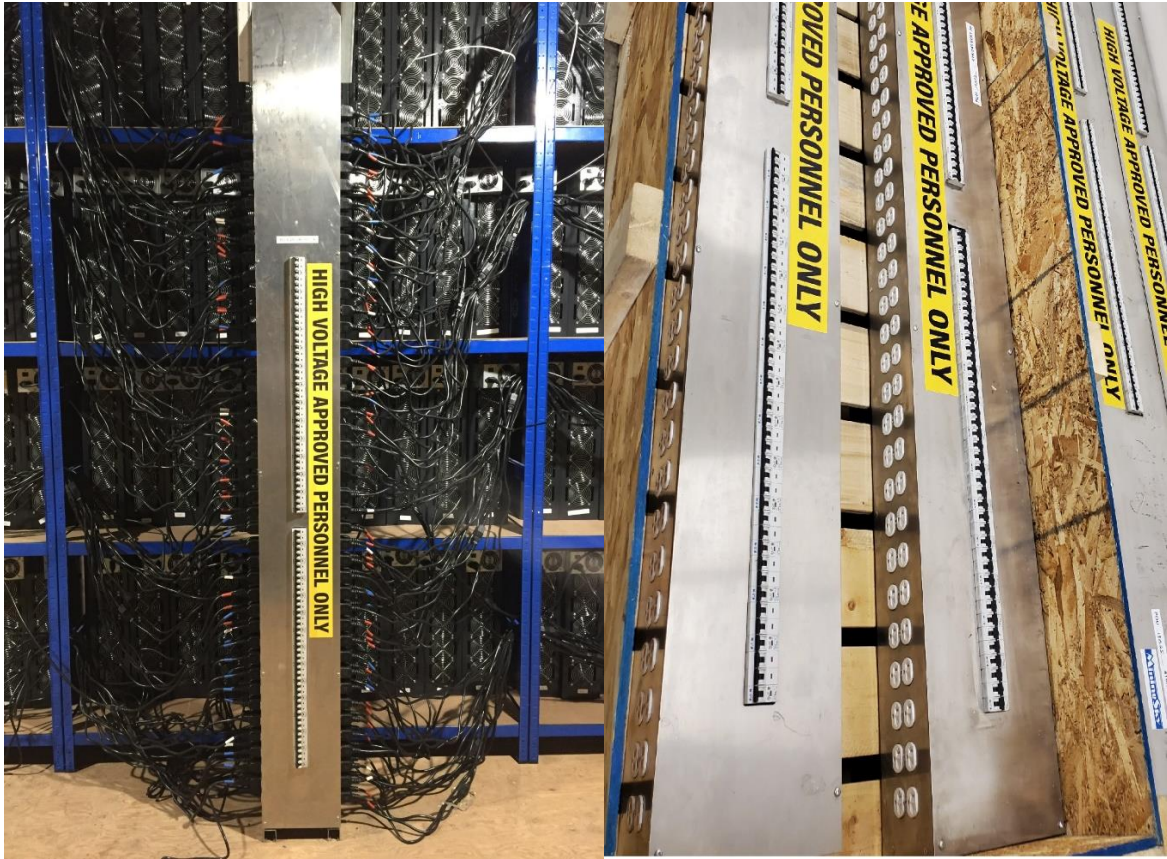
Photo 1: Exterior of the PDU
